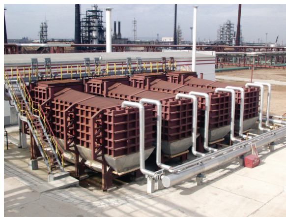
Fig. 6. Hermetic sedimentation tanks in the system of circulating water supply of the oil refinery
