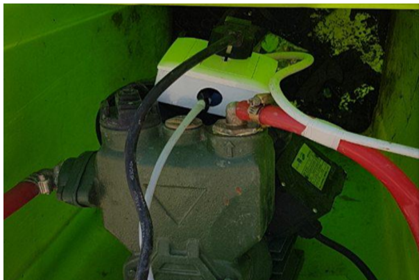
Fig. 4. The cleaning system pump connected to the relay
