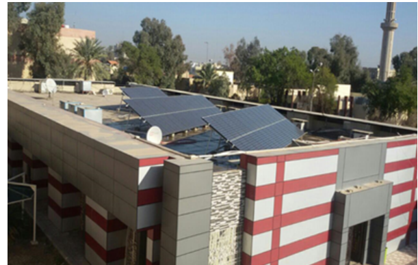
Fig. 1. The 15 kW PV solar system
