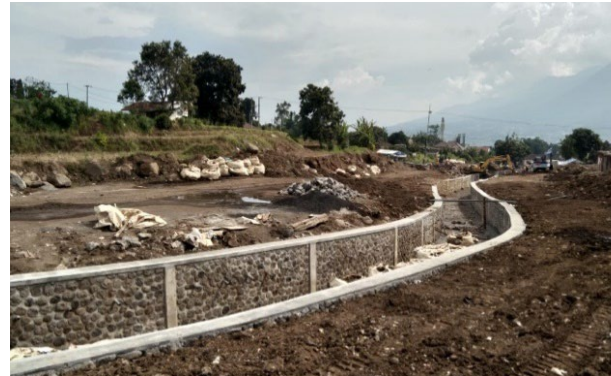
Fig. 3. The repair process of the river body around the tourist destination of Mount Pucung Adventure Park, Batu City (source: researcher documentation, 2022)
