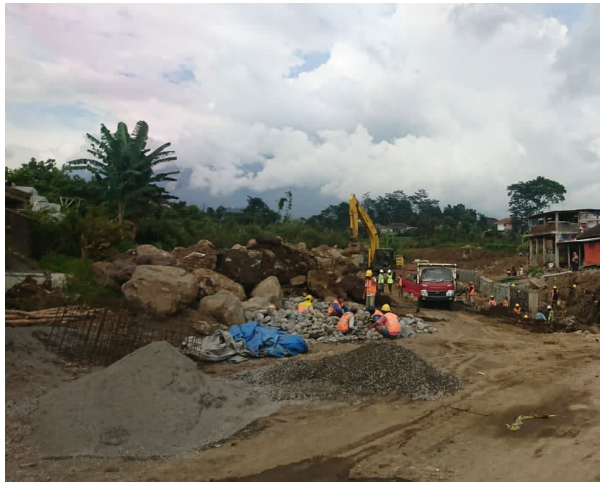
Fig. 2. The bridge is the main access to the Gunung Pucung Adventure Park, Batu City which was damaged due to flash floods (source: researcher documentation, 2022)
