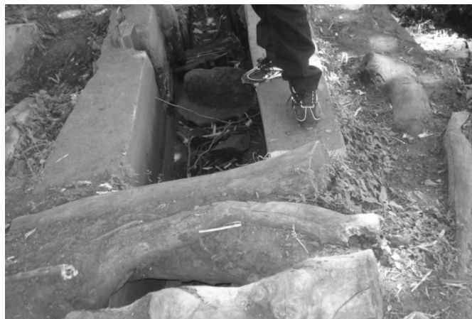
Fig. 8. Canal crossing made from abandoned log, flow obstruction in Argeda SSI
